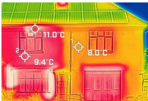
From the outside: Left half is solid brick – losing heat fastest; right side is insulated cavity wall.
